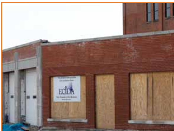
Vacant Seneca Street gas station undergoing adaptive reuse to become retail site to serve Larkin District workers and residents.
